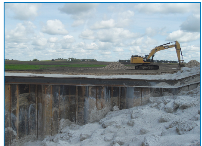
Construction underway at a CREP wetland located in the Boone River watershed
