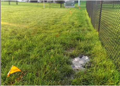
Lack of water infiltration
