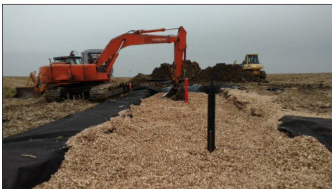
Bioreactor installed in Keokuk County
