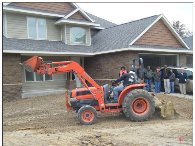
A contractor demonstrates the soil quality restoration practice of deep tillage on a compacted urban lot at a Rainscaper certification training.
