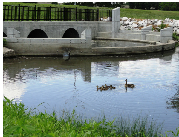
This multi-tiered outlet structure on the forebay installed above DMACC Lake traps sediment, allowing easy cleanout and lake protection.
