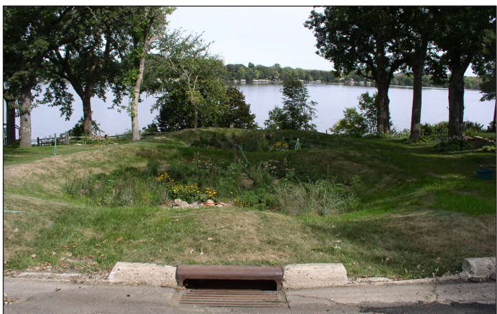
East Okoboji Lake is visible in the background of this multi-tiered bioretention cell that is cleansing street water before discharging it to the lake.
