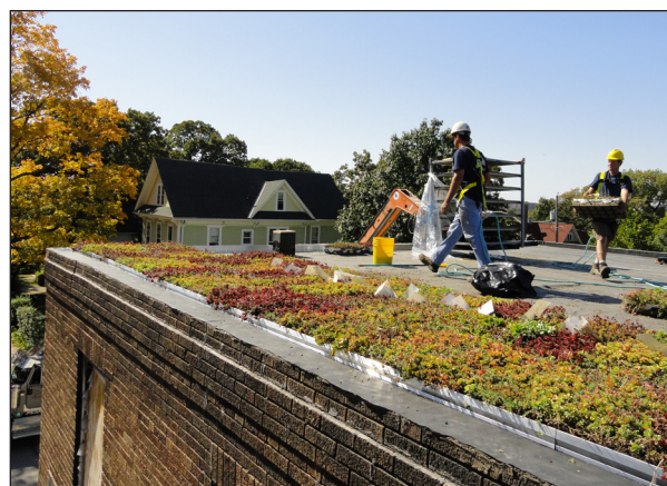
This green roof is part of a building renovation in Des Moines that features a treatment train of stormwater management practices.
