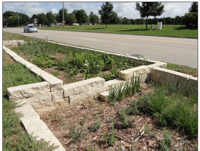
A bioretention project in Ankeny's Summerbrook Park treats street runoff to protect Fourmile Creek and demonstrates how to rainscape.
