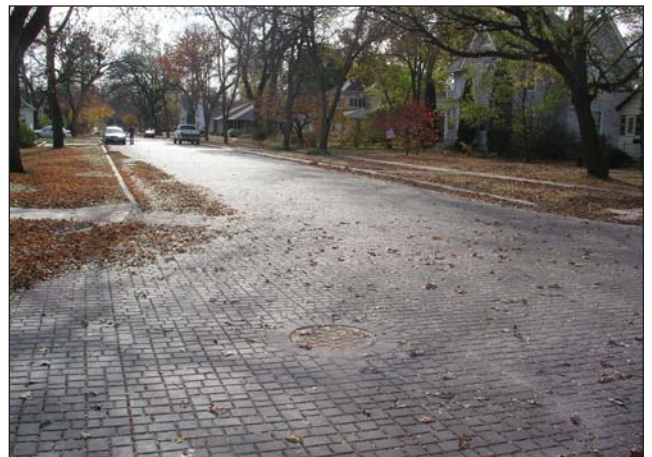
Charles City installed 17 blocks of permeable pavement. This is believed to be the largest street renovation using permeable pavers in the Midwest. This project eliminated street flooding and the need for storm sewer upgrades while enhancing neighborhood property values.
