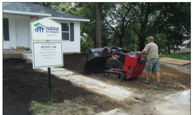
Compost is incorporated by Delf's Landscaping as part of a soil quality restoration demonstration at a Habitat for Humanities project in Davenport. Aunt Rhodies Landscaping also installed a rain garden. Financial assistance came from a grant through Iowa American Water. Fourteen additional projects resulted from this demonstration.
