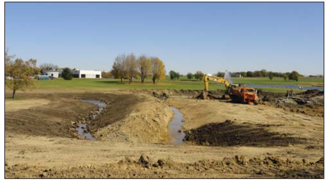
A stormwater wetland being installed adjacent to DMACC Lake where a large storm drain previously released untreated runoff. The runoff works its way through the long pathway of the constructed wetland system where it will have time for many pollutants to be removed through natural processes.
