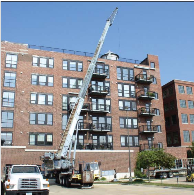
A crane lifts pallets of plants to the roof of Water Tower Place in downtown Cedar Rapids, where a green roof was installed.
